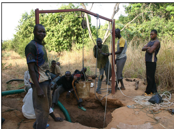
Working as a team; each with his role. (Norm turned the I beam so it looks like it is supposed to be bent!)
